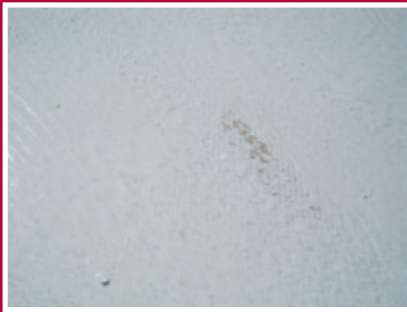
Before applying GacoFlex S-20 the existing roof had significant deterioration
