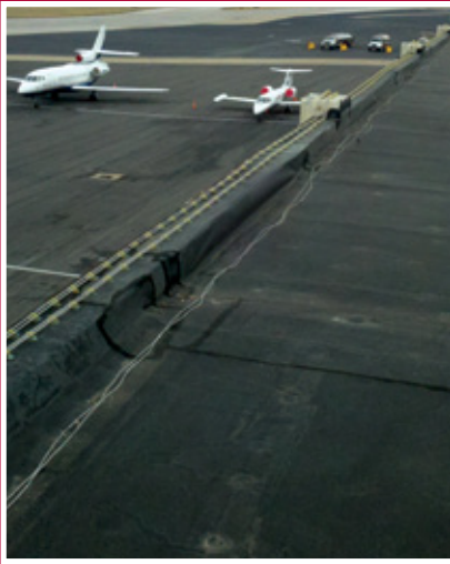
Before applying GacoFlex S-20 the existing roof had significant deterioration
